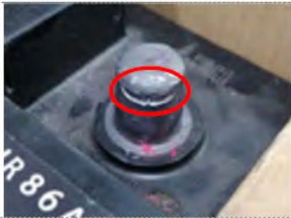
Damaged battery (-) pole
