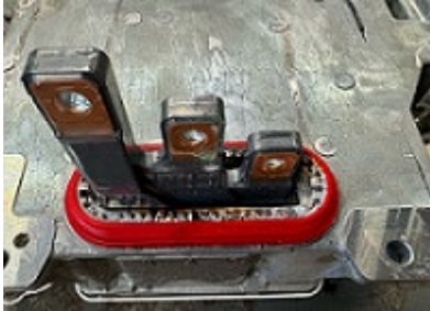
Figure 4: Corrosion on high-voltage system connection for power and control electronics for electric drive.
