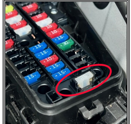
No Good (not secured)
