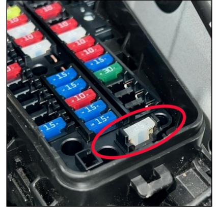
No Good (not secured)
