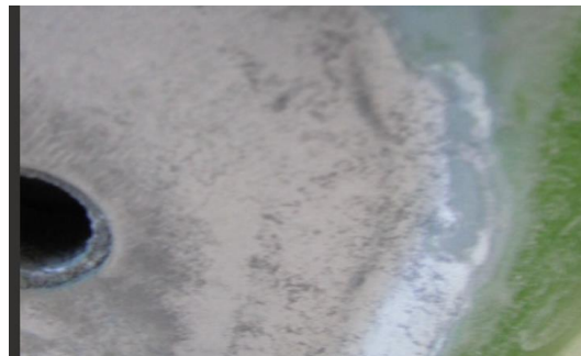
Pitting Found After Sanding Example (Fig. 1)
