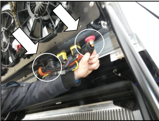
Figure 3: Radiator fan drive, main power cable connections at radiator side
