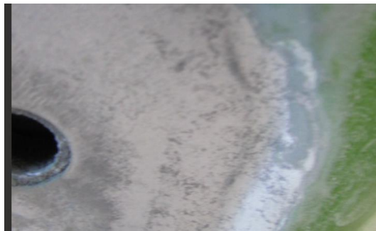
Pitting Found After Sanding Example (Fig. 1)
