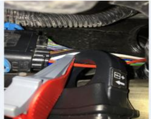
Figure 9: power supply wiring to the air suspension compressor.
