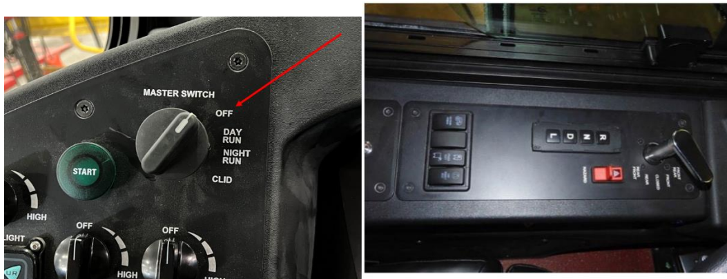
Master Switch Off, Hazards Off
