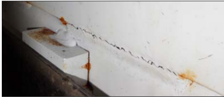
Figure 4 — Example of Weld Cracking
