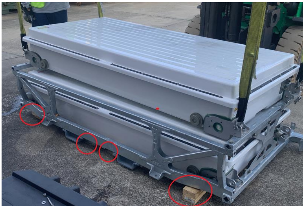
Figure 12: ESS battery packs wooden block under the assembly reference.
