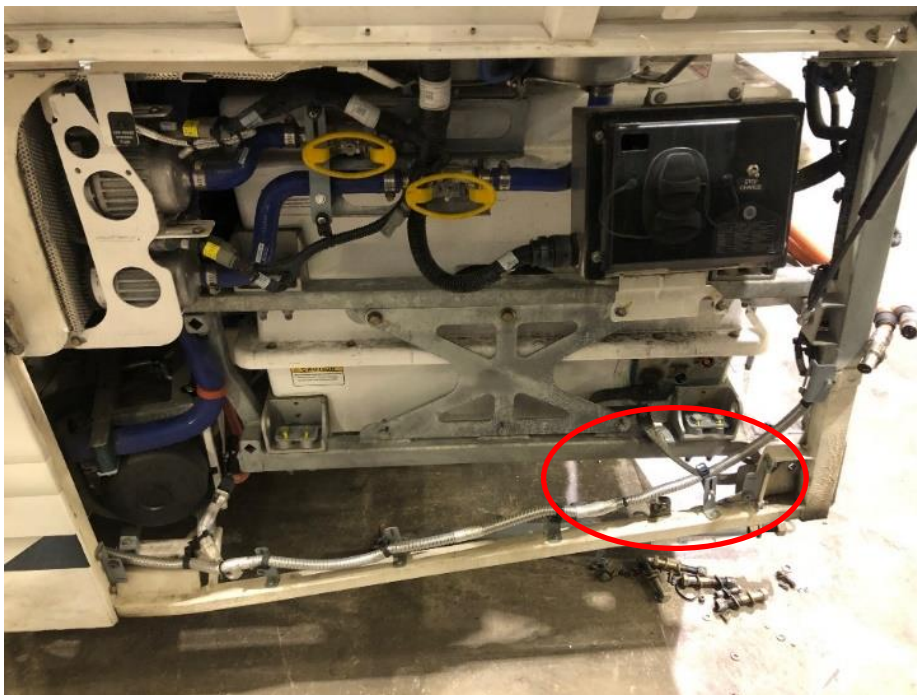
Figure 4: ESS ground strap to bus frame location reference.
