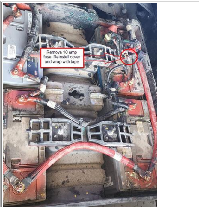
Figure 12: Auxiliary Battery Box - Fuse Removal
