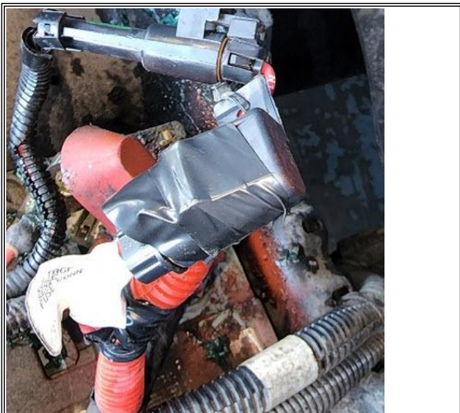
Figure 13: Fuse Holder - Fuse Removed, Cap Taped with Electrical Tape
