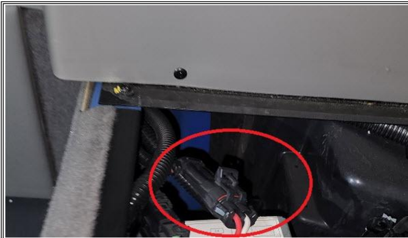
Figure 2: 100B/C No-Idle System controller power sense/ground connector
