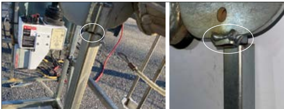
Figure 8 — Examples of Cracking in the Vertical Cross-Member
