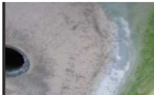
Pitting Found After Sanding Example (Fig. 1)
