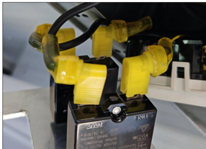
Figure 3 — 15/20 Amp Circuit Breaker With Incorrectly Crimped Terminal Pins
