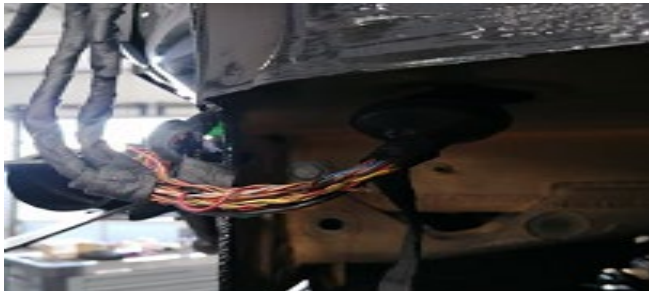
Figure 2: Wiring beneath the wrapping.
