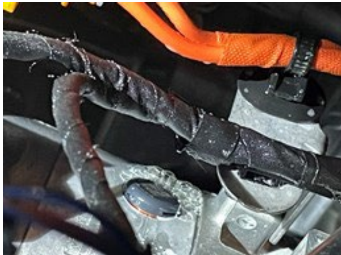
Figure 2. Active compressor pressure relief valve leak.
