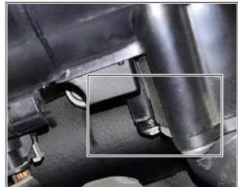
Slight traces of coolant (current type of coolant regulator with a leakage tank)
