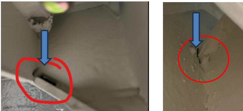
FIGURE 2: SHOWN VIEW OF MISSING WELD – INSPECT TO SEE IF ALL WELDS COMPLETE (MISSING WELD NEAR END)
