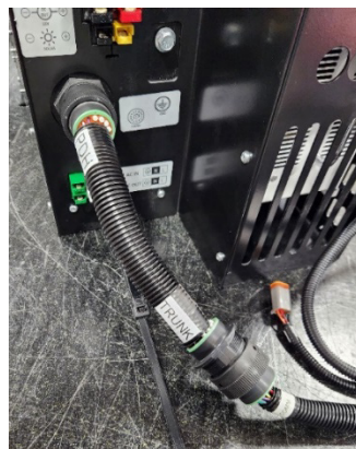
Figure 5. Finished installation of AC detect harness
