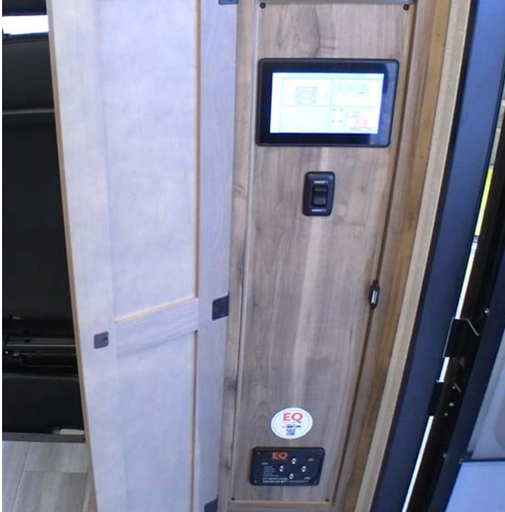
Cabinet where the G12 is located
