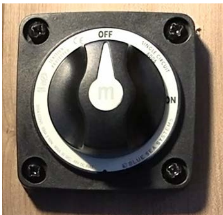
Coach Main 12 VDC Shutoff switch
