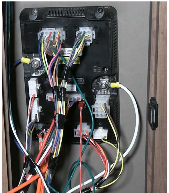
G12 Panel mounted inside wall
