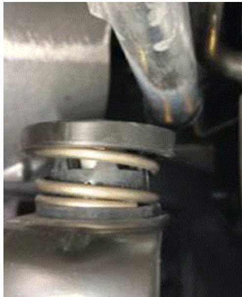
Figure 10. Correctly seated compressor isolator / spring assembly.
