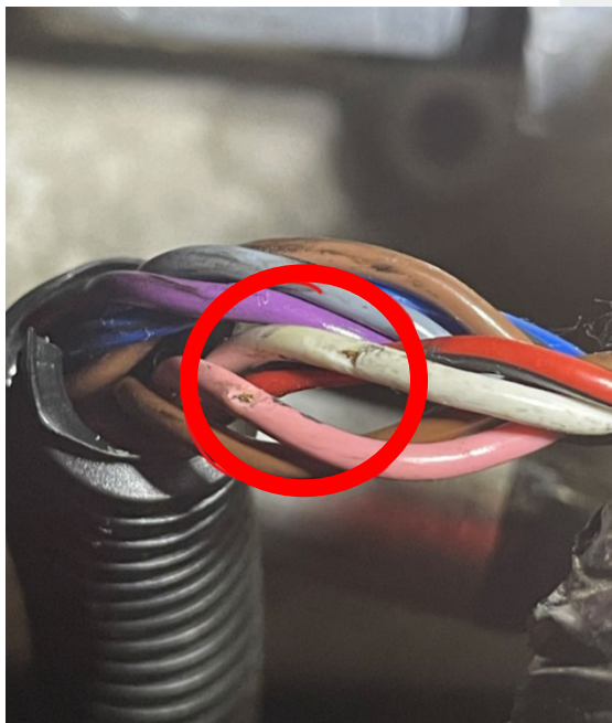
Figure 13 – Evidence of damage observed (1 of 2)
