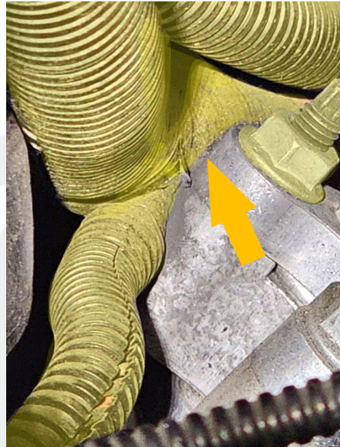
Figure 12 – Evidence of rubbing observed (2 of 2)
