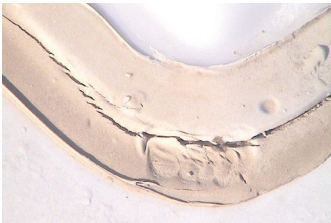
Traditional industry roof sealant showing common problematic cracking.
