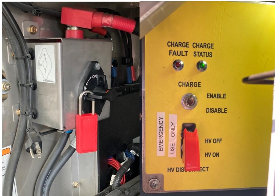
Figure 1: Lockout tagout location reference
