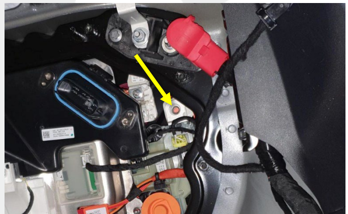
Figure 4 — Positive DC link busbar bolt missing
