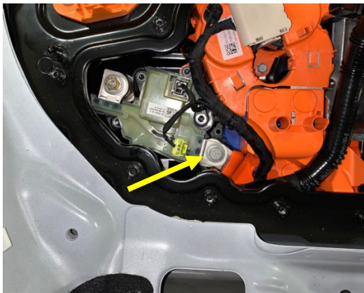
Figure 1 — Negative DC link busbar bolt present
