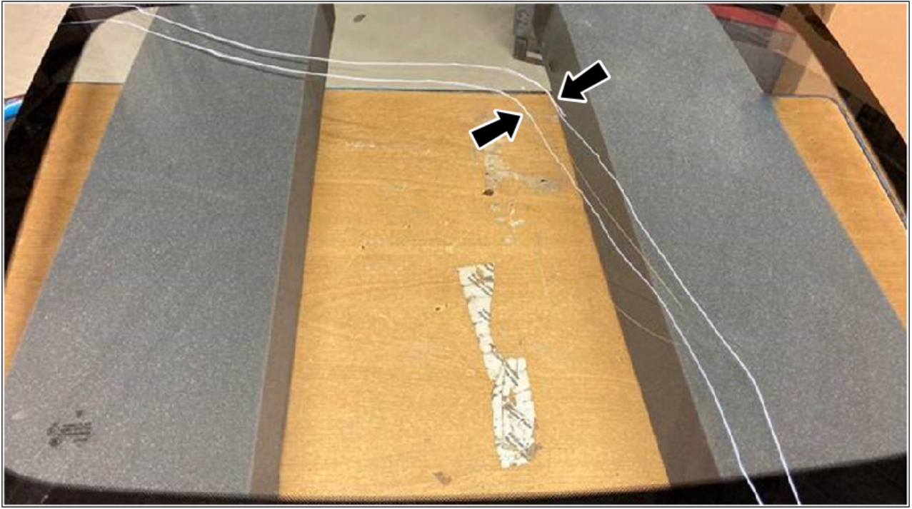
Marked crack pattern (example illustration on a Cayman GT4 RS rear window)
