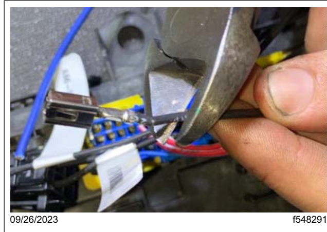
Fig. 23, Cutting Off the Terminal
