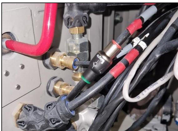
Figure 1: In compartment ahead of left front wheel, location of additional single-check valve (= new situation)
