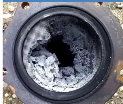
Eroded and broken Catalyst
