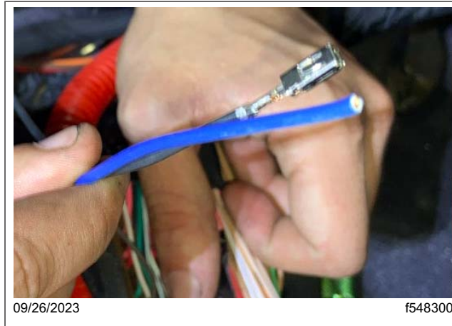
Fig. 32, Wire Removed from Cavity 6 of the SSAM X2 Connector and the Shorter Blue Wire, to be Spliced Together
