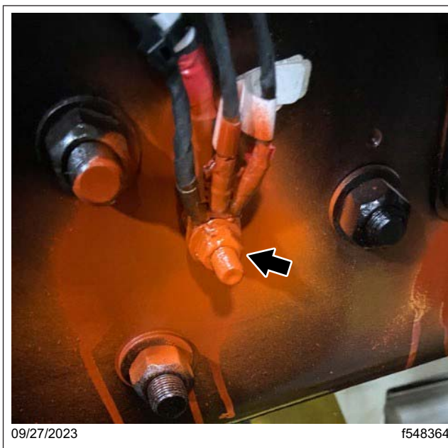
Fig. 96, Ground Stud Coated with Red insulating Epoxy
