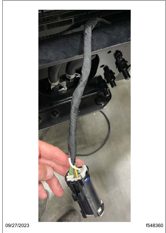
Fig. 92, Exposed Wiring Wrapped with Fabric Tape
