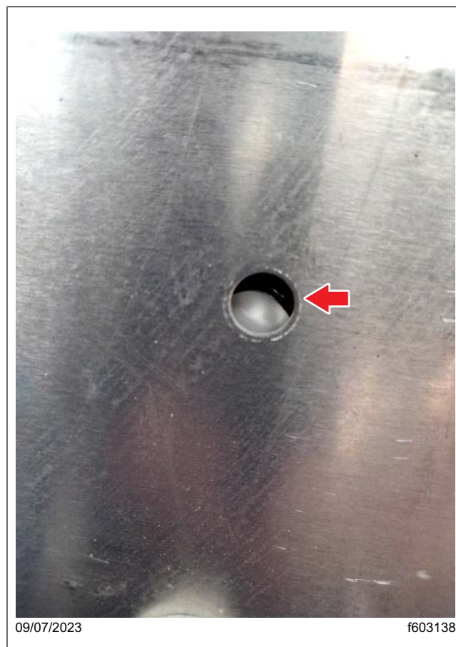
Fig. 10, Misaligned Floor Panel Toe Kick Edge Hole with the Front Wall Hole
