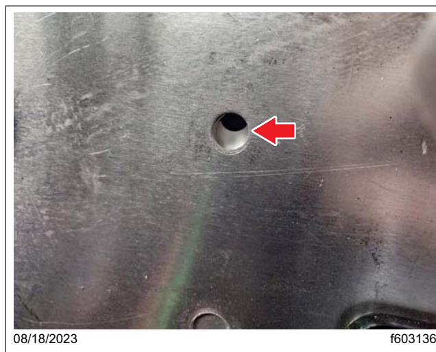
Fig. 8, Misaligned Panel that needs to be Drilled
