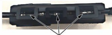
Exposed slice visible.
