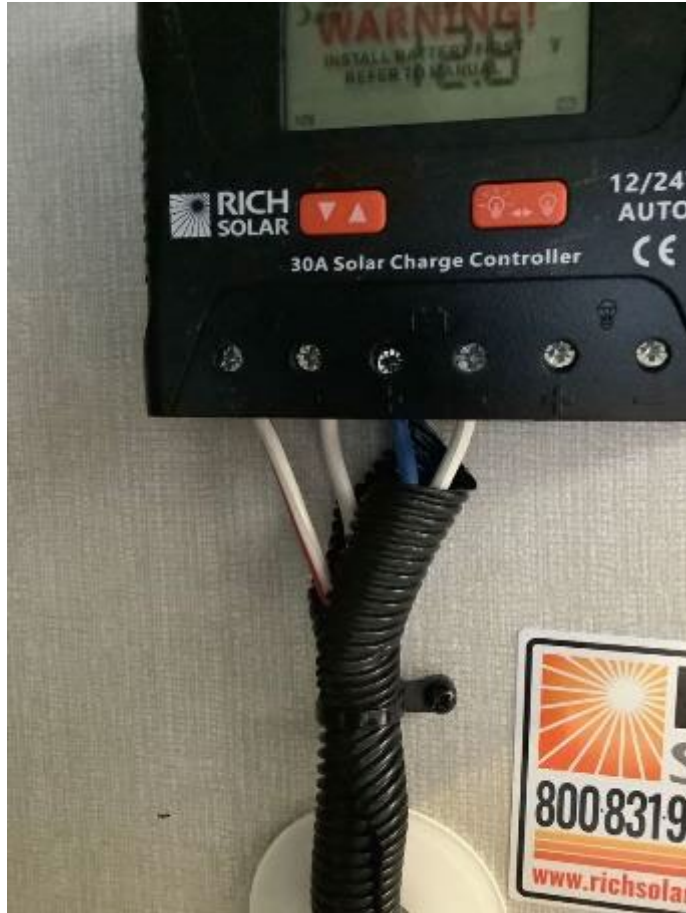
FIGURE 1 – INCORRECTLY WIRED SOLAR CONTROLLER
