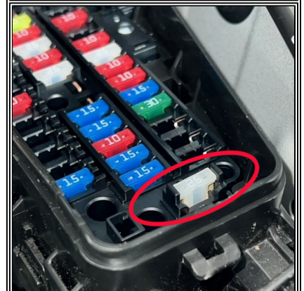
No Good (not secured)
