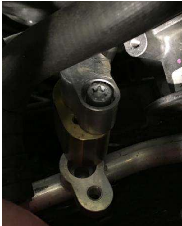
Figure 14. Location and connection of the adaptors for the rear unit A/C lines
