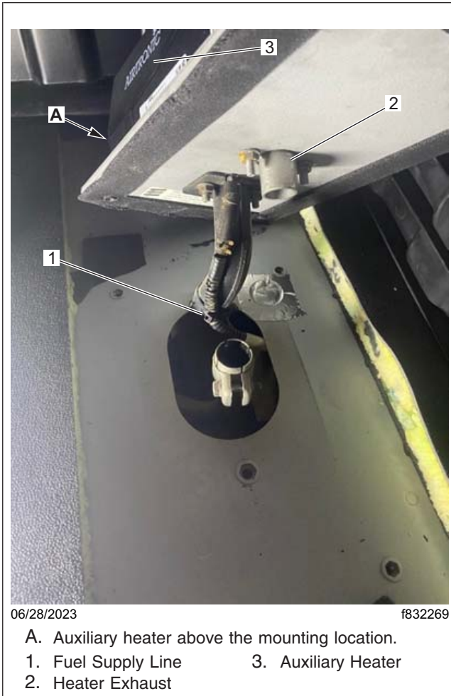
Fig. 23, Location of the Auxiliary Heater Fuel Supply Line
