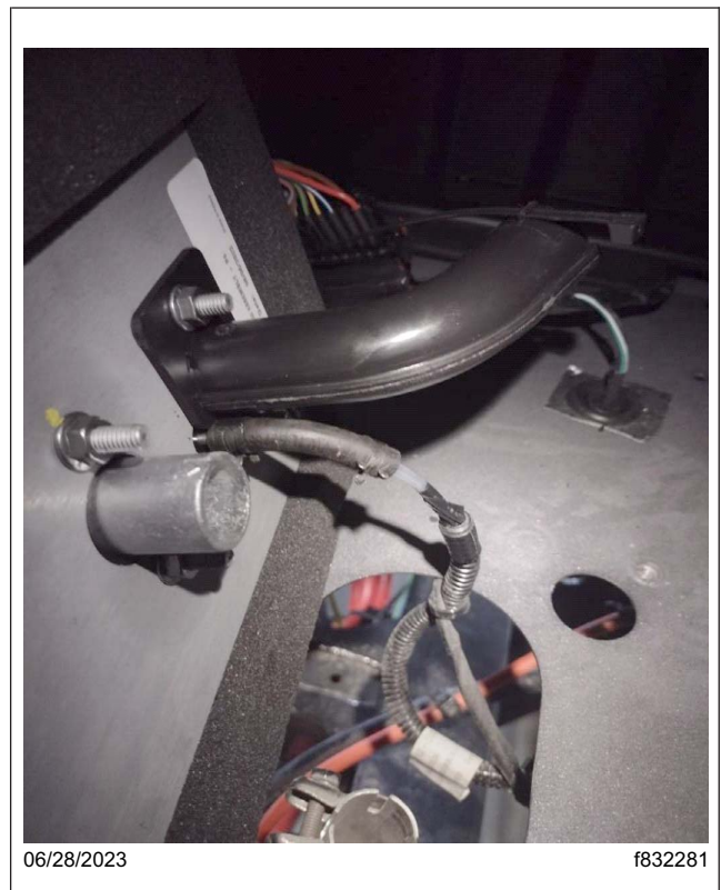
Fig. 26, Fuel Line Connected to the Heater
