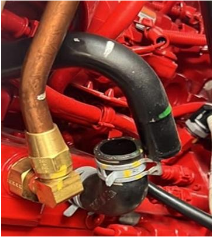
Figure #1: CAC to Air Compressor Intake hose separated
