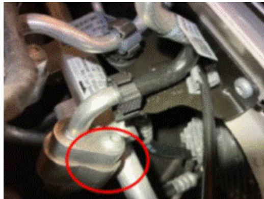
Figure 11. Service port mounting interference with adjacent line.
