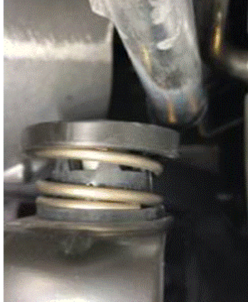
Figure 10. Correctly seated compressor isolator / spring assembly.
