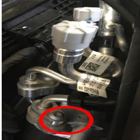
Figure 3. The refrigerant lines are making contact.
