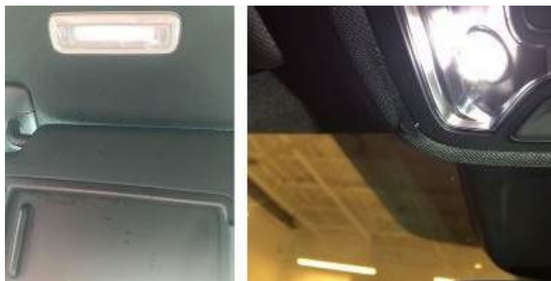
Figure 1. Water intrusion near the headliner.
