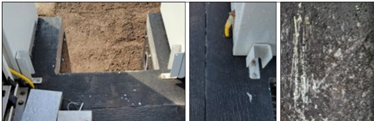
Figure 2 — Examples of Normal Wear and Damage
