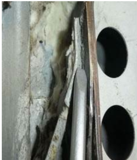
Figure 16. Incorrect engagement of the chisel end.
