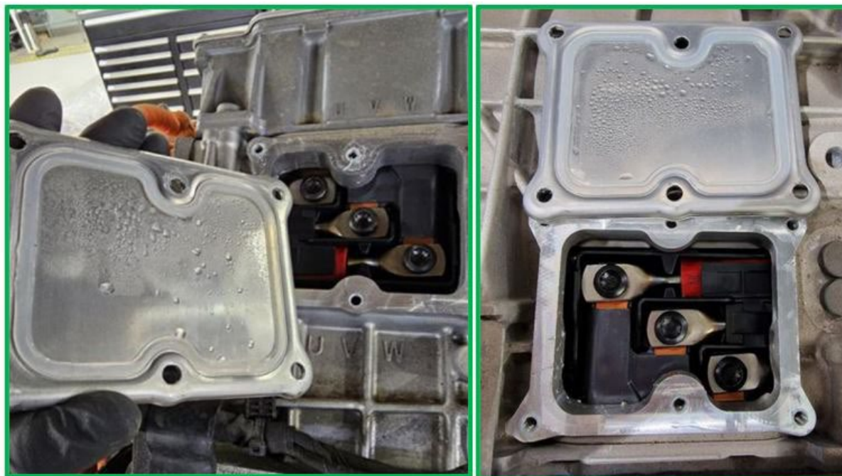
Figure 1. Condensation on the cover of power electronics connections.
