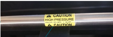
A CAUTION HIGH PRESSURE CNG FUEL LINE, p/n 10600076
