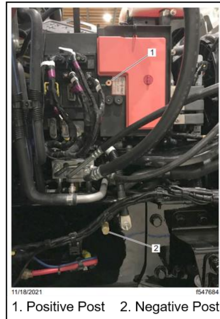
Fig. 5, Positive and Negative Posts on the Electric Vehicle Distribution Module (EVDM)
