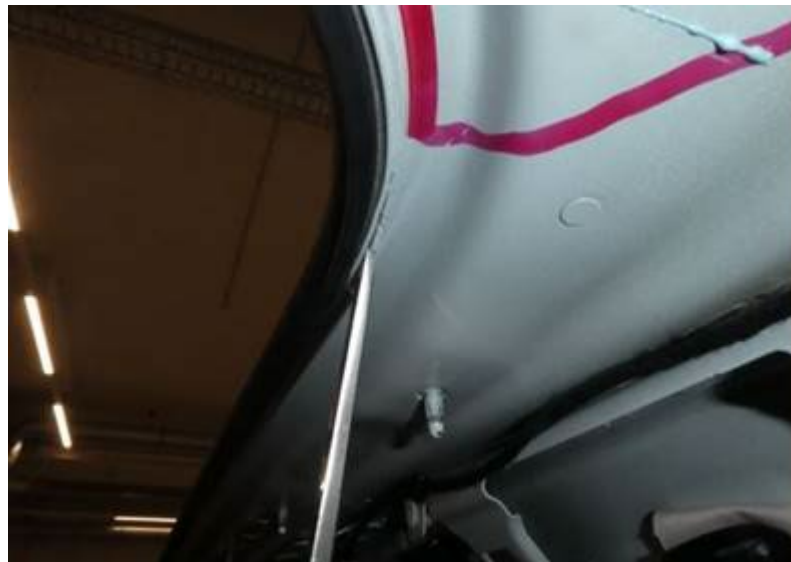
Figure 7. Adhesive joint separated.
