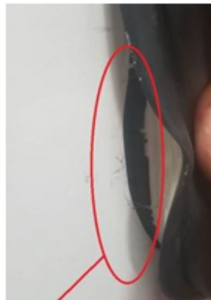
FIGURE 10 POOR BUTYL ADHESION TO WALL
