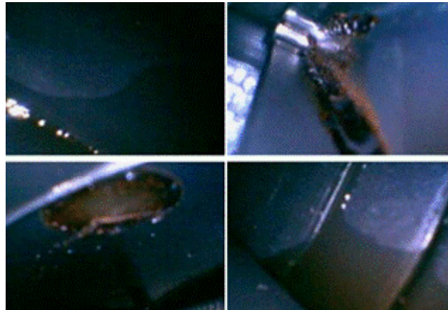
Figure 6. Borescope images showing evidence of water intrusion into the fresh air blower housing.
