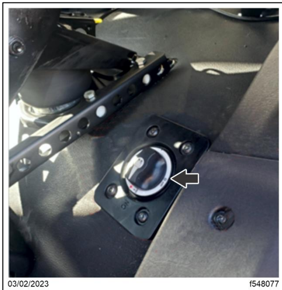
Fig. 1, Battery Disconnect Switch under the Driver's Seat
