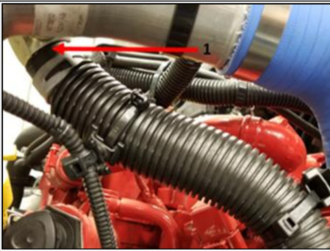
Figure 2: Air Compressor Inlet Hose
